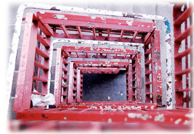
Figure 9: Degeneration; Park Hill Flats Sheffield
